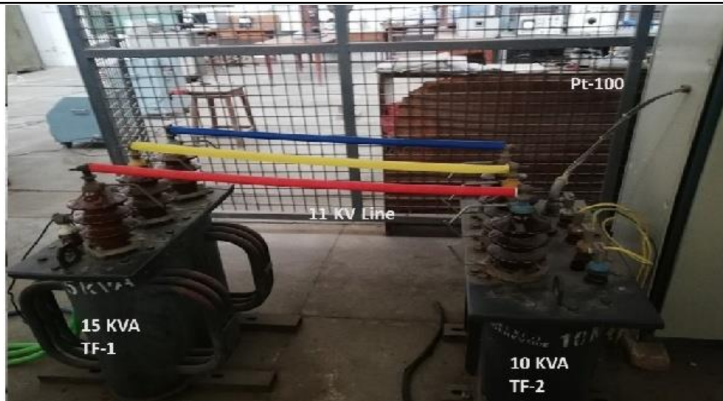
Fig. 2: Transformers for laboratory setup
